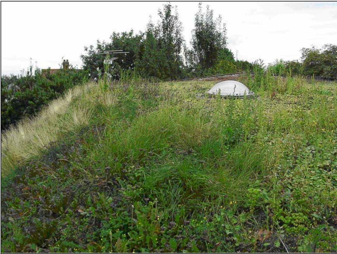
Figure 1: Part of the main roof at 11 Shaw's Cottages, south London (photo by the author).
