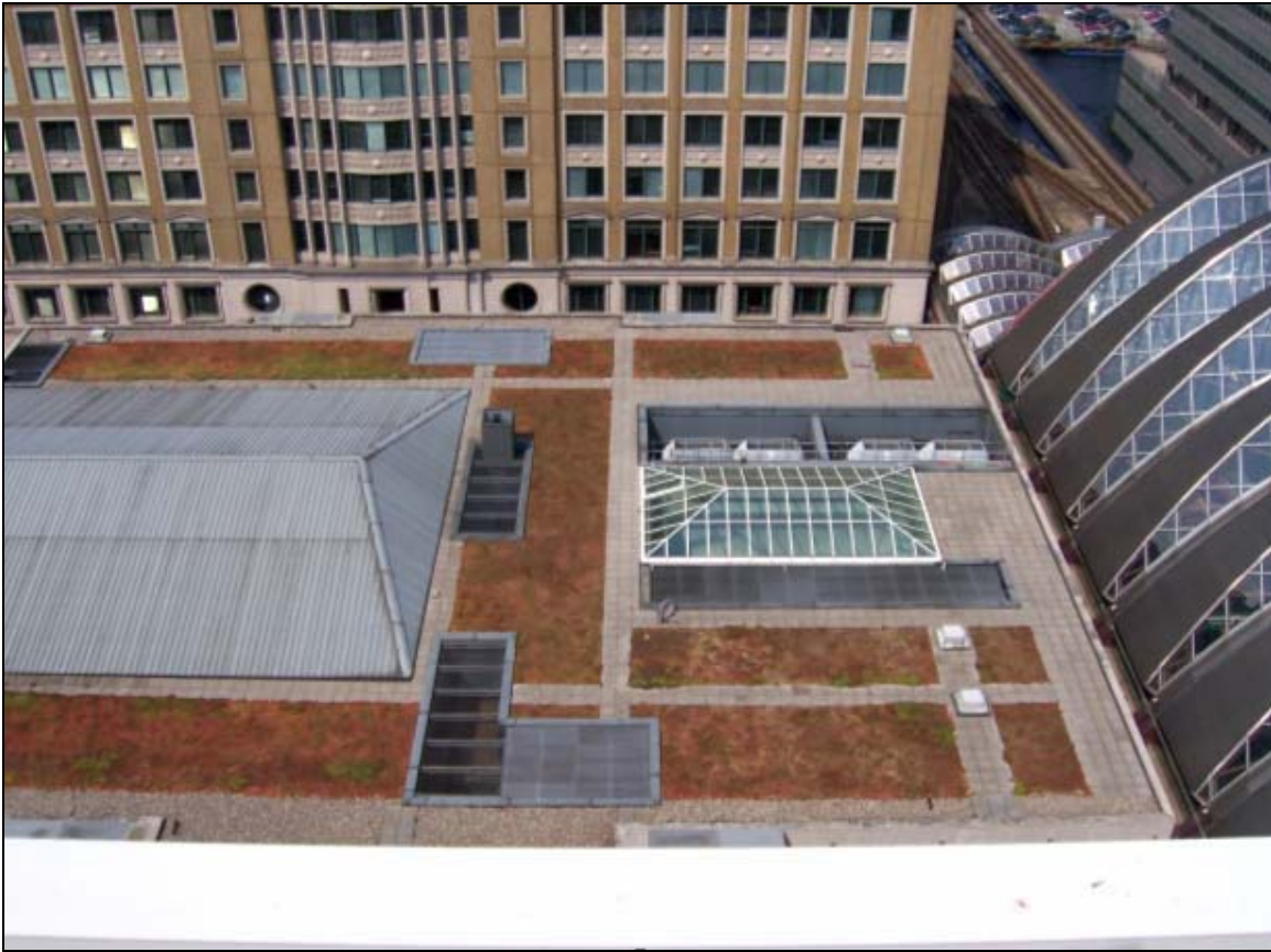
Figure 3. Sedum roof on Retail Building, Canary Wharf, east London (photo by the author).
