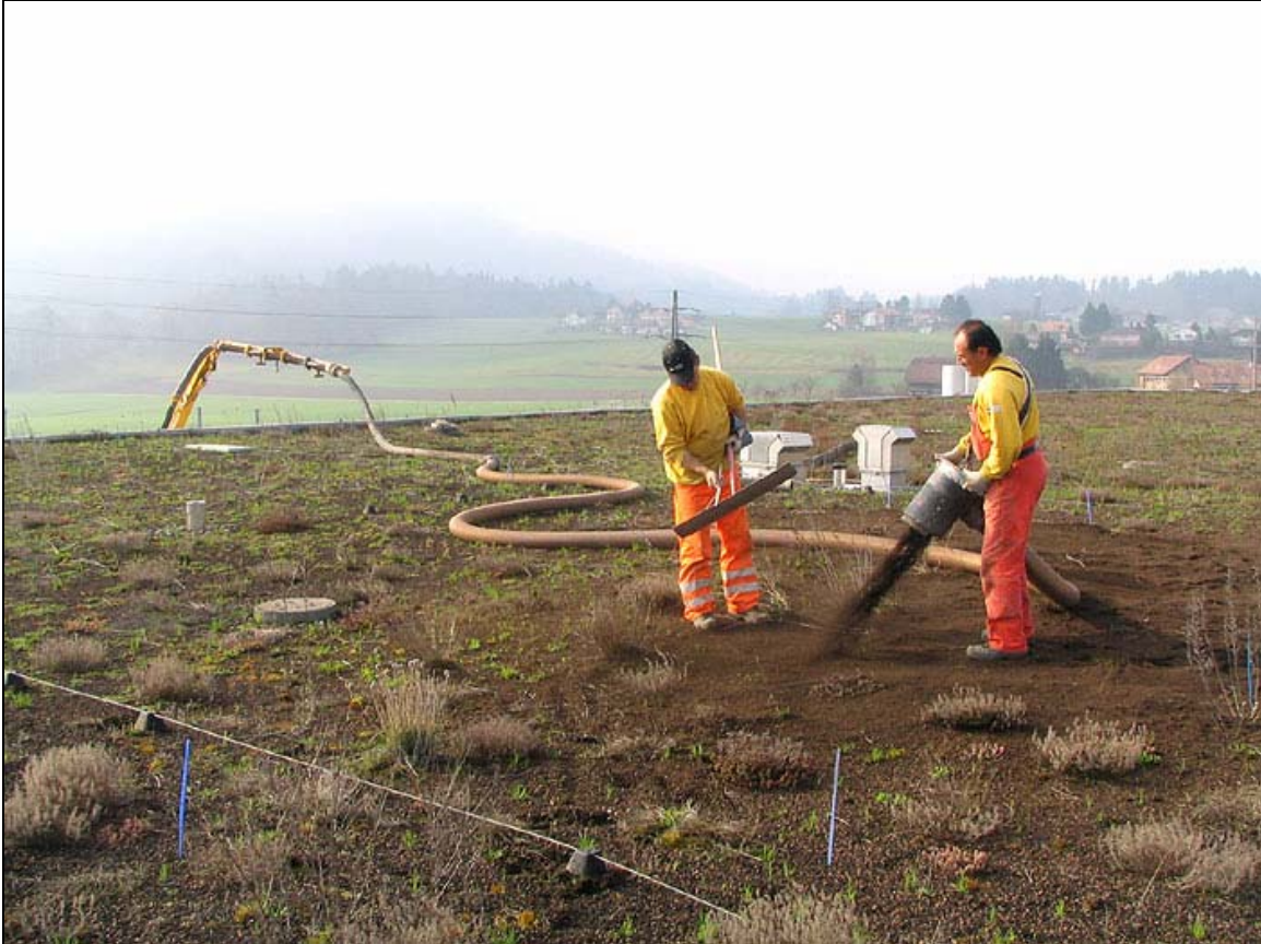
Figure 1: Project workers add compost substrate (about 4 cm) to the topsoil of the roof at Shoppyland, Berne. (Photo by N. Baumann)
